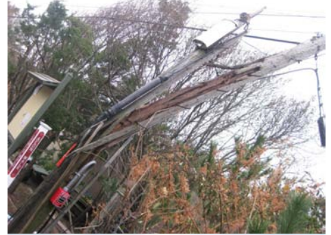
Broken electric pole at Aeon and Lewis...
